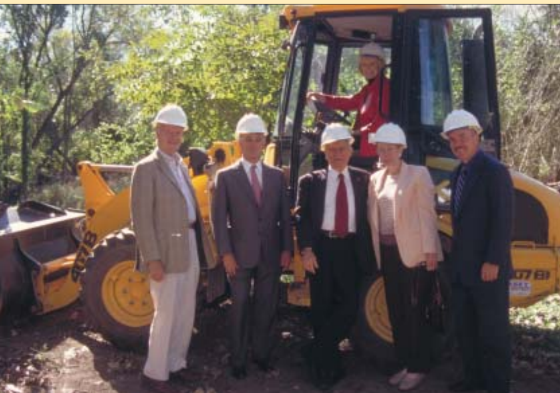
▲ Brookfield Zoo broke ground this year on a spacious new Wolf Woods habitat, made possible by generous support from The Regenstein Foundation. On hand for the start of construction were (left to right) Chicago Zoological Society representatives Trustee Philip W.K. Sweet, Chairman Edward McCormick Blair, Jr., and President Dr. George Rabb, and from The Regenstein Foundation, Chairman Susan Regenstein Frank (seated), Secretary Joan Gorsuch, and Vice President Tom Staszak.
